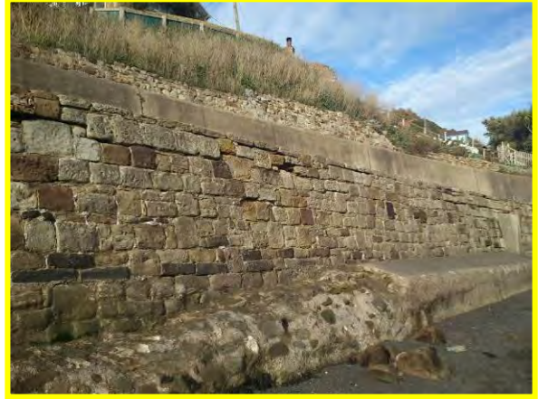
Gaps at joints and missing blocks, Oct 2012. (Asset Ref. 1221D901D0601C03)
