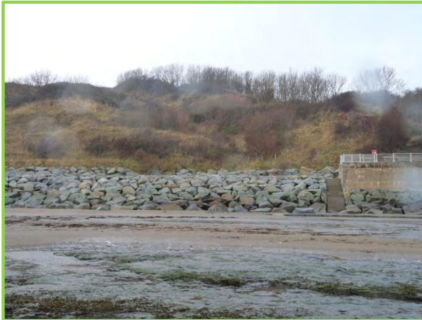
MU17/1 No change was noted to this unit following the December 2013 storm surge.
