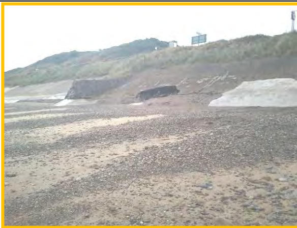
Large void in revetment adjacent to recent patch repair, Oct 2012. (Asset Ref. 1221D901D0702C02)
