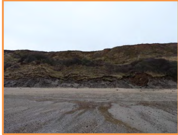
MU29/AF – Extensive toe erosion throughout unit. Note particularly severe toe erosion on left of photograph. December 2013 (Partly Active).
