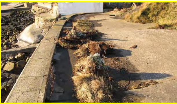
Promenade on top of northern seawall, 17 th December 2013. Evidence of overtopping shown. (Asset Ref. 1221D901D0601C01)
