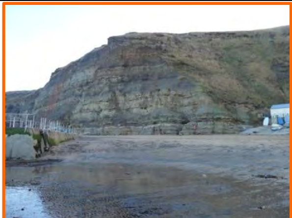
MU4/2 Beach condition post December 2013 storm surge. Note absence of talus at base of cliff. (Partly Active)
