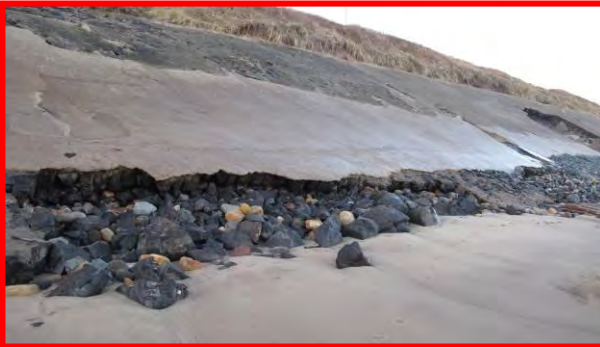
Extensive damage to toe of revetment, 17 th December 2013. (Asset Ref. 1221D901D0702C02)
