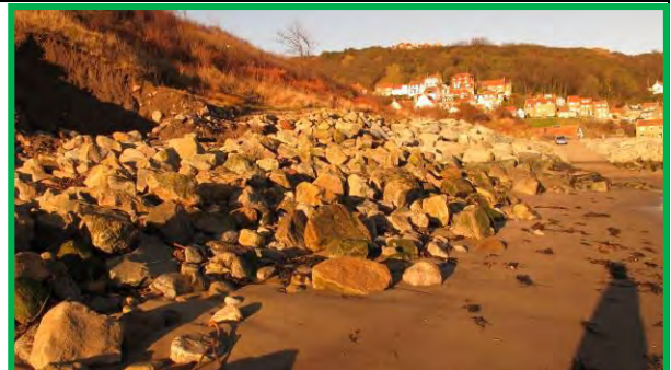
Southern end of Runswick Bay rock armour defences, 17 th December 2013. (Asset Ref. 1221D901D0602C01)
