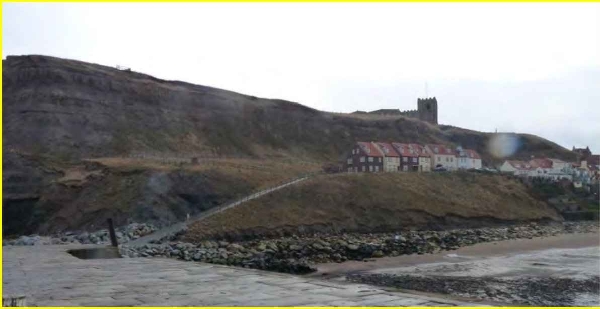
MU12/1 Note toe erosion above rock armour along full length of the slope. December 2013
