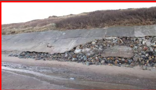
Extensive damage to revetment temporarily filled in, 17 th December 2013. (Asset Ref. 1221D901D0702C02)
