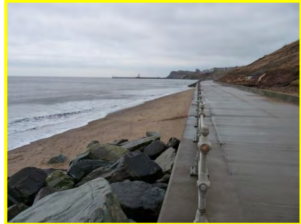
MU11/1 – Gap in rock armour beneath active lower slope December 2013. (Locally Active).
