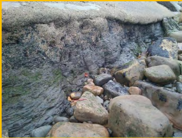
Displaced toe armour, undercutting to concrete revetment and abrasion damage to revetment, Oct 2012. (Asset Ref No.1221D901D0701C02)
