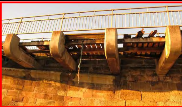
Cantilevered footway, 17 th December 2013, showing storm damage on 5 th December. (Asset Ref. 1221D901D0702C04)
