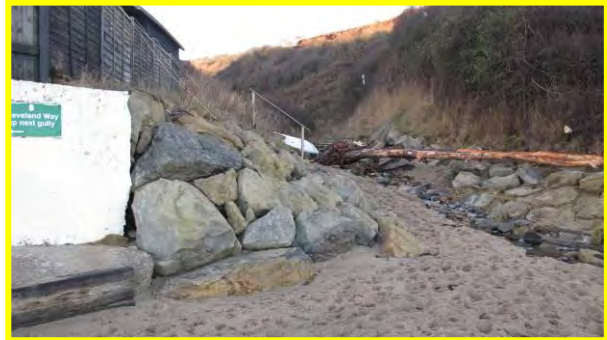
Northern end of defences at Runswick Bay sailing club, 17 th December 2013. Note higher beach levels compared to 2012. (Asset Ref. 1221D901D0602C05)
