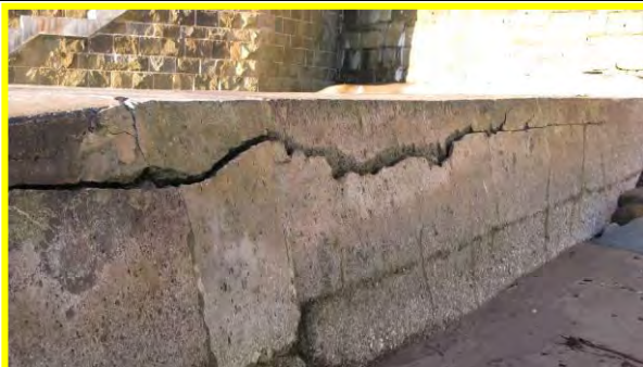
Large horizontal crack to breakwater, 17 th December 2013. (Asset Ref. 1221D901D0601C02)
