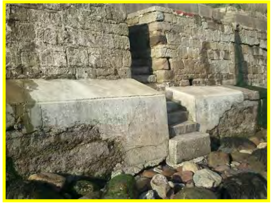
Undercutting of toe adjacent to steps, Oct 2012 (Asset Ref. 1221D901D0601C03)
