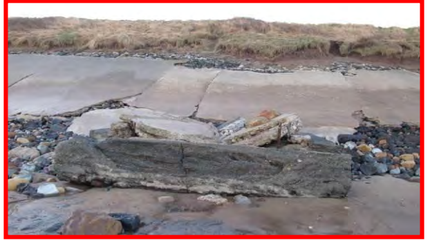
Extensive damage to revetment on 17 th December 2013. Same location as previous photo (left). Again slight recovery of beach sand evident. (Asset Ref. 1221D901D0702C02)
