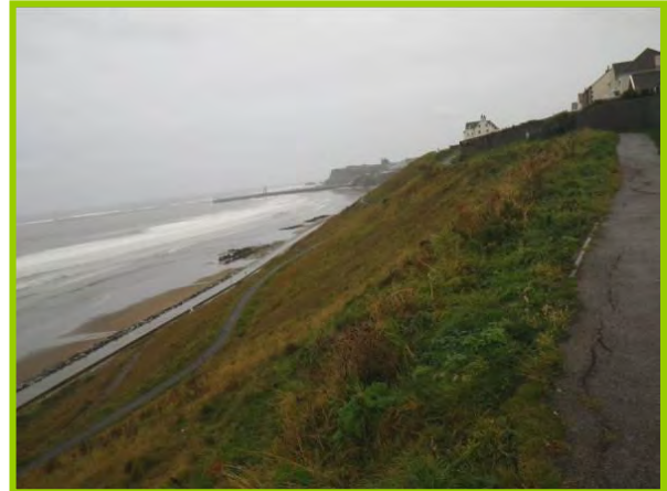
MU11/1 The upper sections of the slopes are in good condition (Inactive) Oct 2012
