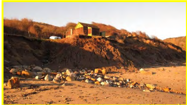
Eroding cliffs at Dunsley Dale near Runswick Bay Sailing club, 17 th December 2013.
