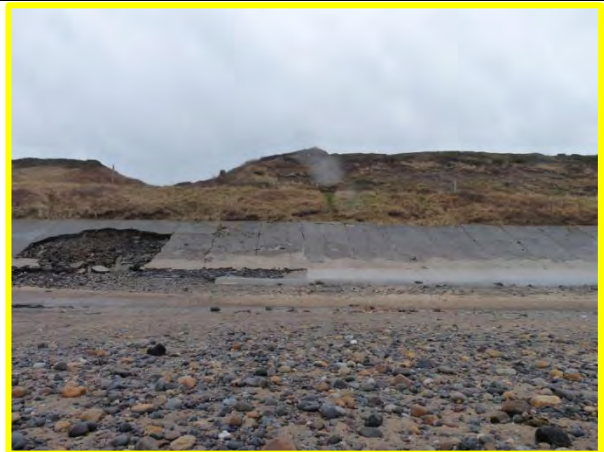
MU9/3 Note erosive features in upper slope and failure of defence at the toe. December 2013
