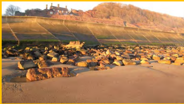
Concrete revetment at the north of Sandsend, 17 th December 2013. (Asset Ref No.1221D901D0701C02)
