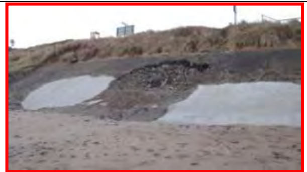
New large void in revetment adjacent to previous and more recent patch repairs, 17 th December 2013. Compare to 2012 inspection (left). (Asset Ref. 1221D901D0702C02)
