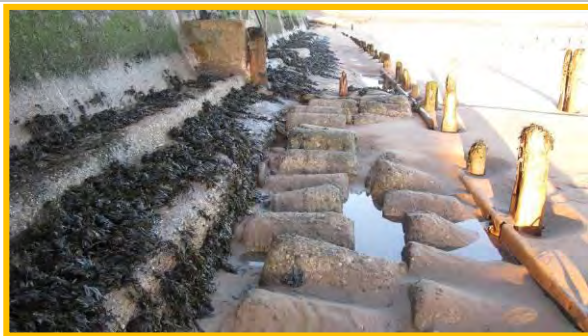
Failed timber groynes and timber breastwork at toe of wall in front of Sandsend, 17 th December 2013. (Asset Ref. 1221D901D0702C01)
