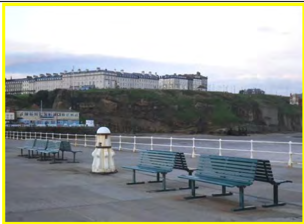
MU11/4 Localised erosion above Whitby Sands (Locally Active)
