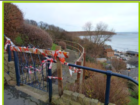
MU28/Y – Cracking in pathway within landscaped gardens Dec 2013
