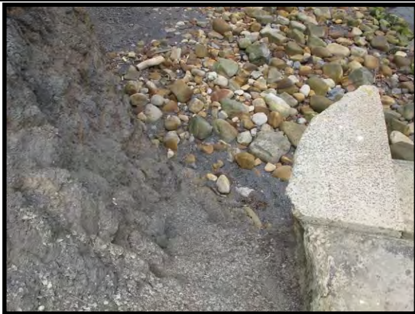
Cliff adjacent to north end of seawall from the top promenade, 10 th July 2013. (Asset Ref. 1221D901D0601C01)
