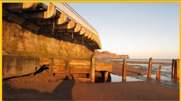
Masonry blockwork sea wall with cantilevered footway, 17 th December 2013, showing larger void under toe apron and failed groynes. (Asset Ref. 1221D901D0702C04)
