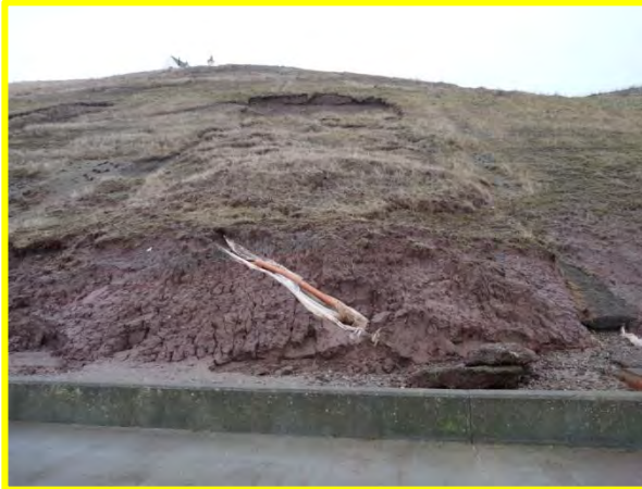
MU11/1 – Reactivation of significant failure in lower slope. Note toe erosion exposing drainage pipe and recently exposed scar. December 2013. (Locally Active)
