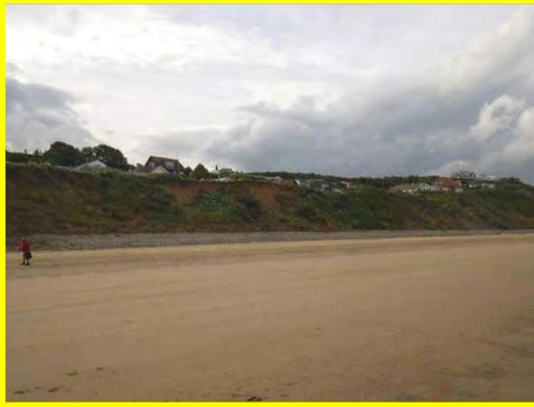
MU29/AR Continuing mudslide activity and toe erosion at Flat Cliffs (Locally Active). Sept 2012
