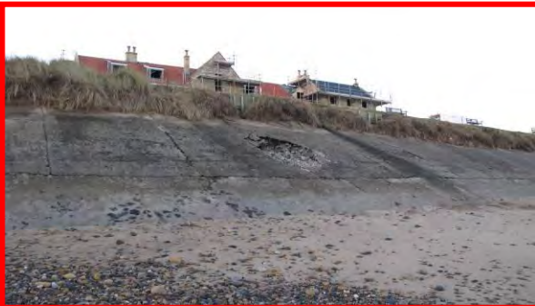
Cracks and voids in surface of concrete revetment, 17 th December 2013. (Asset Ref. 1221D901D0702C02)
