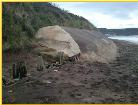
Repair at east end of the concrete revetment since 2009 inspection, Oct 2012. (Asset Ref. 1221D901D0702C02)
