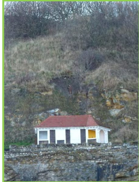
MU22/5 – Small midslope failure (centre photo, above building). December 2013. (Inactive)
