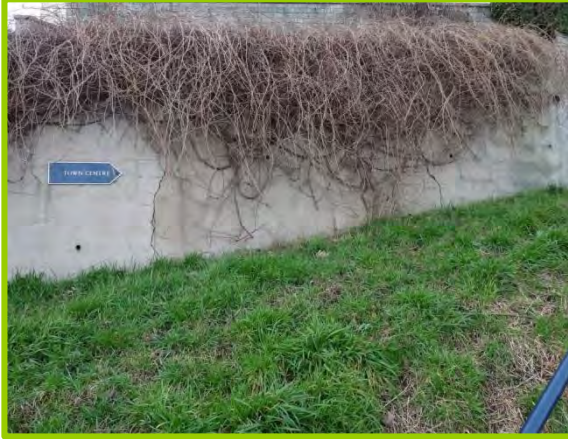
MU27/Y - Cracking in wall in landscaped gardens. December 2013 (Inactive).
