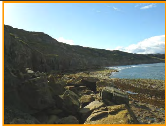
MU23/D1 failed blocks at the toe of the cliff (Partly Active) Sept 2012
