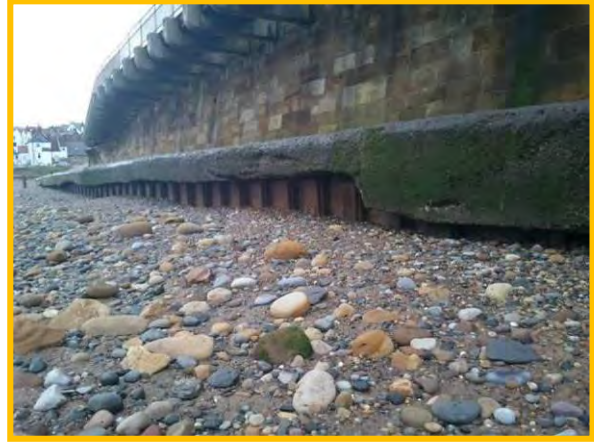
Exposure of toe piling below masonry wall, Oct 2012. (Asset Ref. 1221D901D0702C04)
