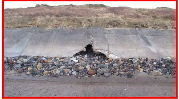
Viewing defence east to west, void in eastern revetment, 17 th December 2013. (Asset Ref. 1221D901D0702C02)
