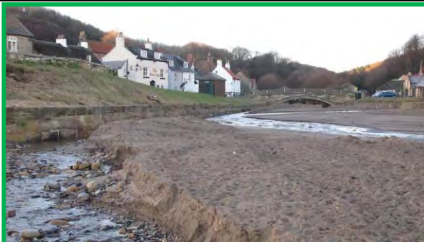
Low masonry wall at East Row Beck, south bank, 17 th December 2013. Note accumulation of sand with the beck cutting through. (Asset Ref. 1221D901D0702C03)
