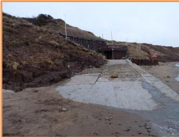
MU27/V – Far northern end of unit. Note encroachment of the toe of the cliff onto the sailing club slipway
