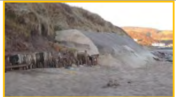
East end of the concrete revetment, 17 th December 2013. Note lower beach levels compared to 2012 inspection (left). (Asset Ref. 1221D901D0702C02)
