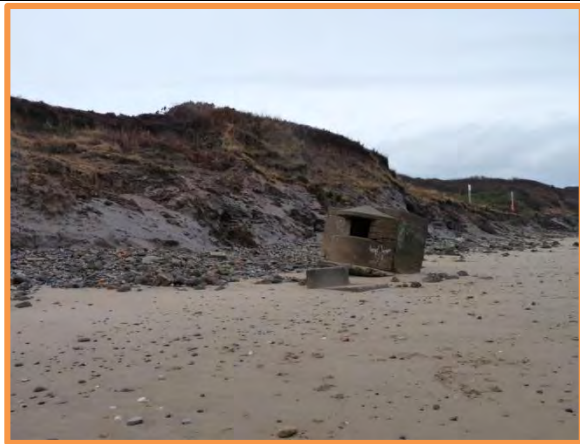
MU29/T – Showing erosion in lower cliff and position of pillbox for future reference. December 2013 (Partly Active).
