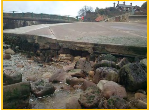
Void under slipway at the north of Sandsend, Oct 2012. (Asset Ref No.1221D901D0701C02)
