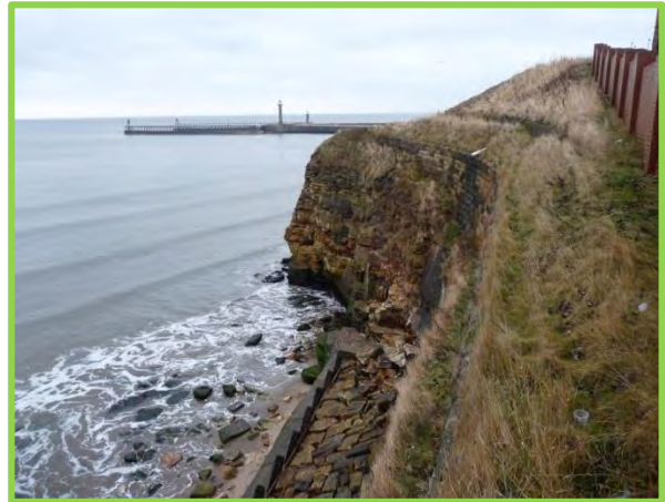
MU11/13 – Small rockfall (centre photo) observed during the post-December 2013 storm surge inspection. (Inactive)
