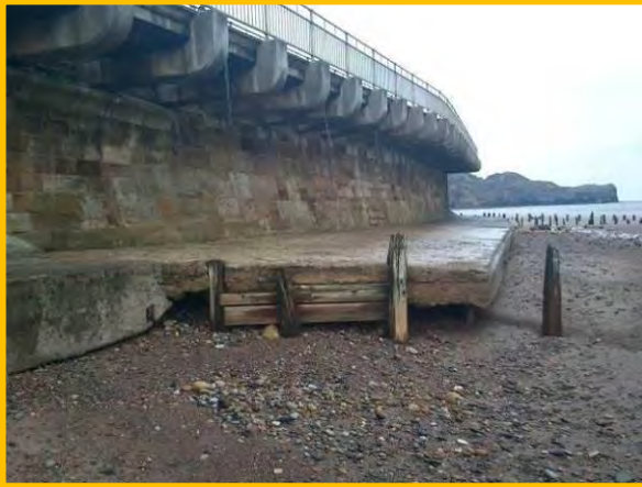
Masonry blockwork sea wall with cantilevered footway, showing large void under toe apron and failed groynes, Oct 2012. (Asset Ref. 1221D901D0702C04)
