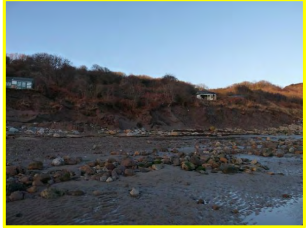
MU7/2 Increased toe erosion at southern end (where defences lower) at far right of photo. Locally Active.
