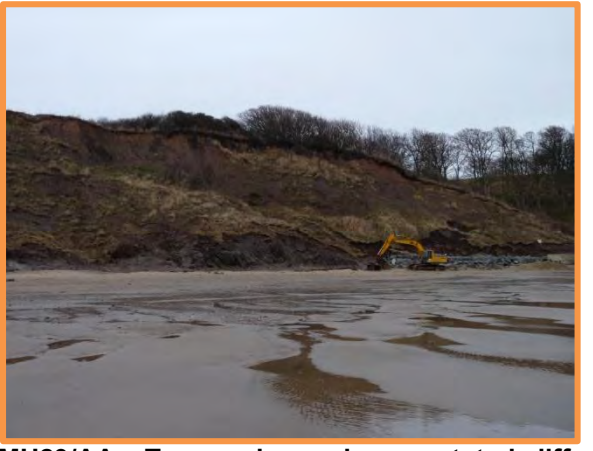
MU29/AA – Toe erosion and unvegetated cliff. December 2013 (Partly Active)
