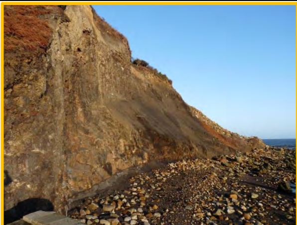
MU6/8 – Small rockfalls witnessed from this unit during post December 2013 Storm Surge Inspection. Partly Active
