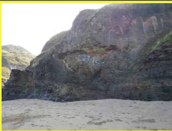
MU7/4 – Toe erosion at the base of the cliff (Locally Active) (September 2012)
