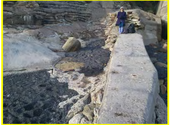
View of northern end of wall with cracked concrete bagwork, Oct 2012. (Asset Ref. 1221D901D0601C06)
