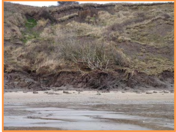
MU29/AC – Further failure of toe. December 2013 (Partly Active).
