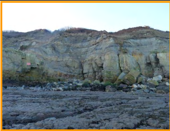
MU23/A – Recent rockfalls (centre right). December 2013 (Partly Active)
