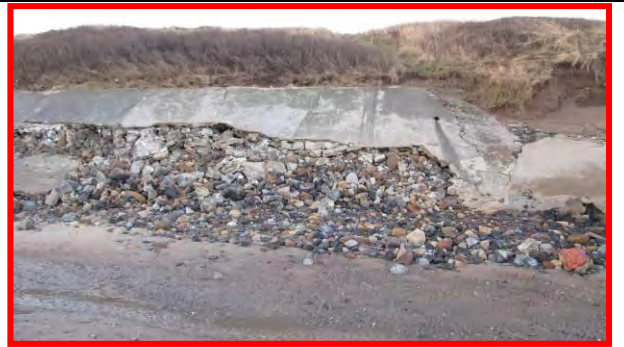
Extensive damage to revetment temporarily filled in, 17 th December 2013. (Asset Ref. 1221D901D0702C02)
