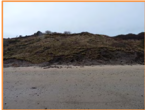
MU29/AH – Still substantially vegetated but with erosion to >2m above the beach at the toe of the slope. Failure affecting near whole slope in left of photo (see photo below). December 2013 (Partly Active).
