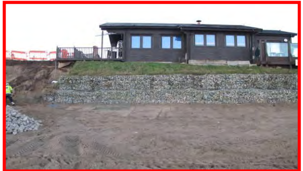
Gabions protecting café at NW end of revetment, 17 th December 2013. Area to the left being repaired with extension to gabions. (Asset Ref. 1221D901D0702C02)
