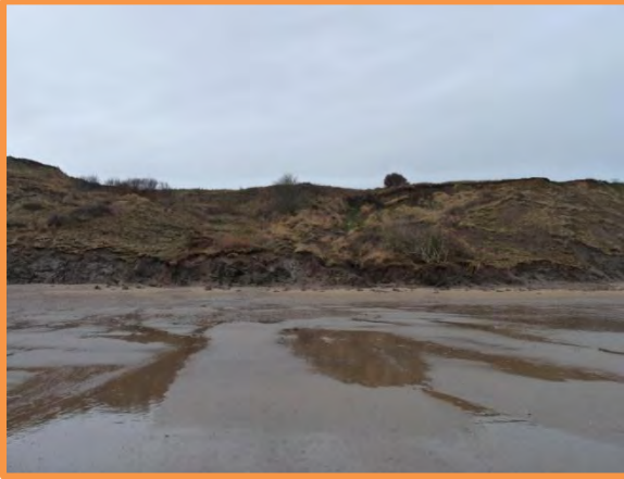
MU29/AC Note further failure of toe to centre left of photo relative to earlier photo (above). December 2013 (Partly Active).
