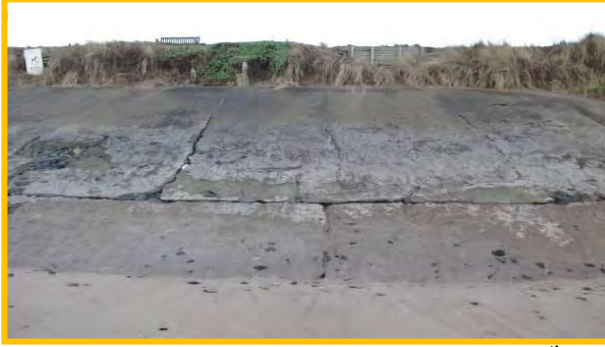
Cracks in surface of concrete revetment, 17 th December 2013. (Asset Ref. 1221D901D0702C02)
