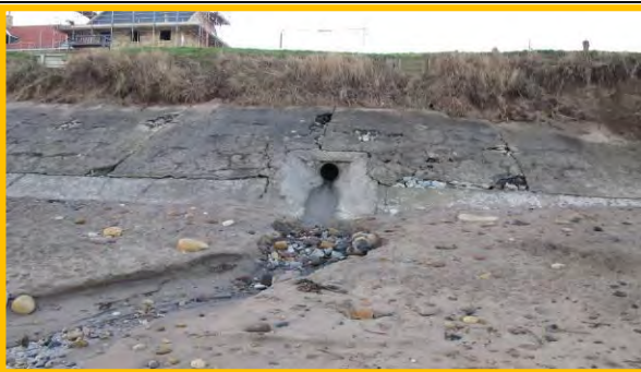
Cracks and voids in surface of concrete revetment, 17 th December 2013. (Asset Ref. 1221D901D0702C02)
