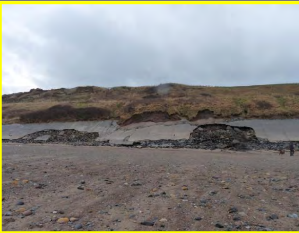
MU9/4 Recent erosion of the toe (above the defences) and erosive features in the upper slopes (December 2013). (Locally Active).
