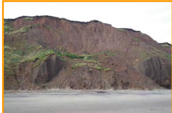
MU10/2 An example of the failures seen along Upgang Beach (Partly Active) (Sept 2013)
