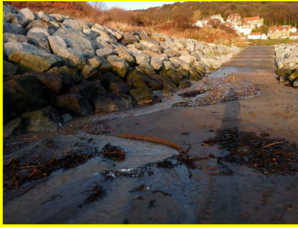
MU7/2 Stream issuing through defences after heavy rainfall during post-December 2013 storm surge inspection. Locally Active.
