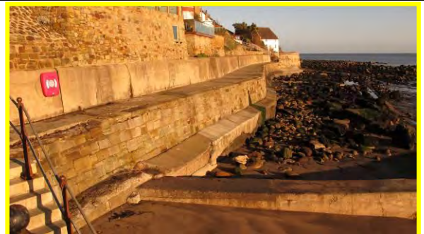
Head of breakwater, 17 th December 2013. (Asset Ref. 1221D901D0601C02) and blockwork wall (Asset Ref. 1221D901D0601C03)
