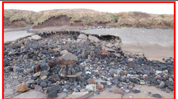
Previous repairs to revetment scoured out, 17 th December 2013. Note slight recovery of beach sand compared to 8 th December photograph at the same location (left). (Asset Ref. 1221D901D0702C02)
