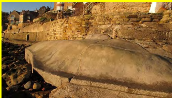
Toe of cottage wall, 17 th December 2013. (Asset Ref. 1221D901D0601C06)
