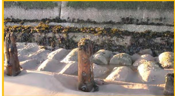
Failed timber breastwork at toe of wall in front of Sandsend, 17 th December 2013. (Asset Ref. 1221D901D0702C01)
