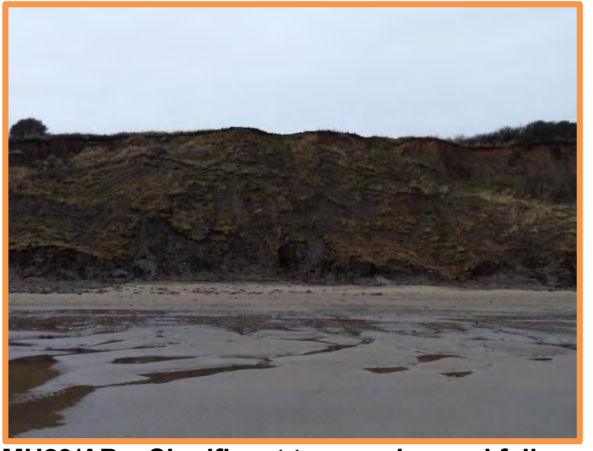
MU29/AB – Significant toe erosion and failure of lower cliff. December 2013 (Partly Active).
