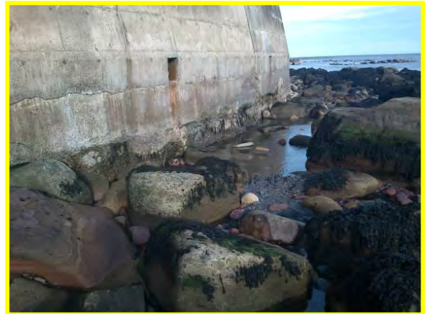
Foreshore scour at toe of seawall, photo from 30/10/2012 (Asset Ref. 1221D901D0601C01) October 2012
