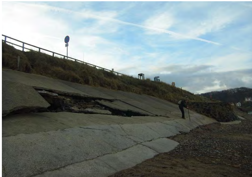
Damage to the defence close to Profile 1dWB1. Photo taken on 9th December 2013
