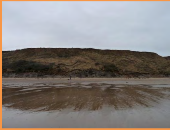
MU29/AE – Toe erosion throughout unit to several metres above the beach level. Note detachment of vegetation indicating failure of lower slope throughout much of the unit. December 2013 (Partly Active)
