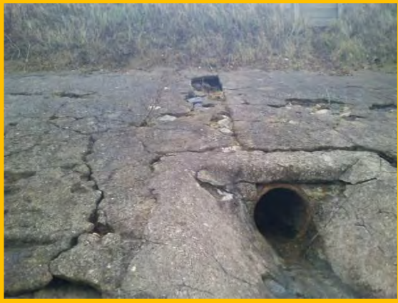
Cracks and voids in surface of concrete revetment, Oct 2012. (Asset Ref. 1221D901D0702C02)
