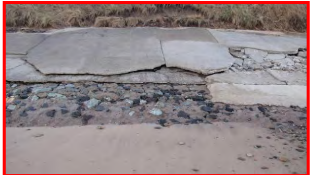
Extensive damage to revetment slabs, 17 th December 2013. (Asset Ref. 1221D901D0702C02)
