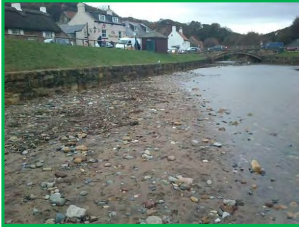
Low masonry wall at east Row Beck, south bank, Oct 2012. (Asset Ref. 1221D901D0702C03)
