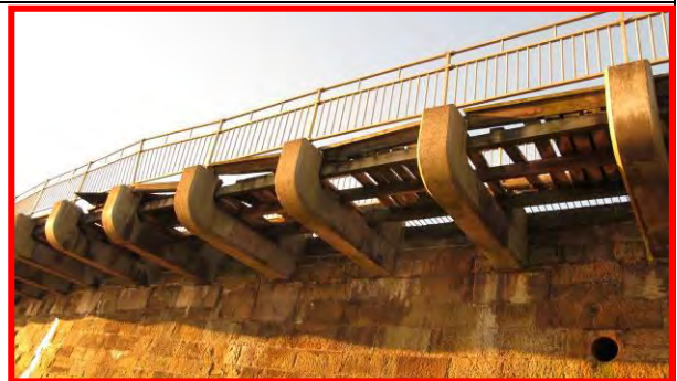
Cantilevered footway, 17 th December 2013, showing storm damage on 5 th December. (Asset Ref. 1221D901D0702C04)
