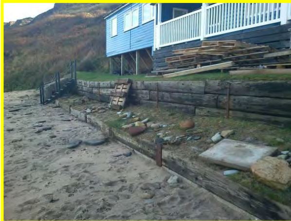
Runswick Bay sailing club timber defences at south end, Oct 2012. (Asset Ref. 1221D901D0602C05)
