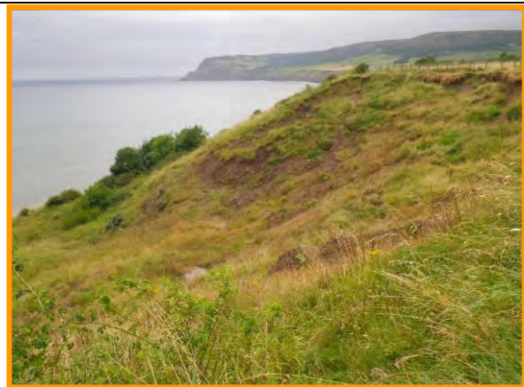
MU17/2 The slope is showing evidence of ground movement (Partly Active). Sept 2012
