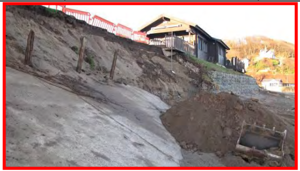
Corner of gabions protecting café at NW end of revetment being repaired, 17 th December 2013. (Asset Ref. 1221D901D0702C02)
