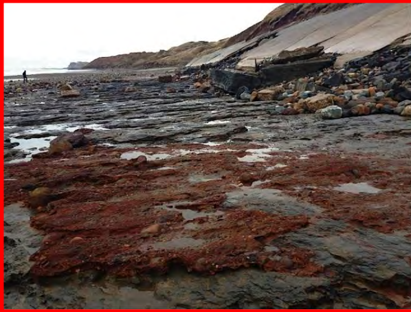
Sandsend seawall revetment and eroded beach following the storm surge of 5 th December 2013. Photo taken on 8 th December 2013, NYCC inspection. (Asset Ref. 1221D901D0702C02)
