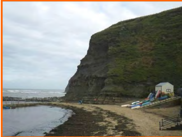
MU4/2 –Vegetated cliff with localised erosion, behind Staithes harbour (Partly Active). Photo from Sept 2012
