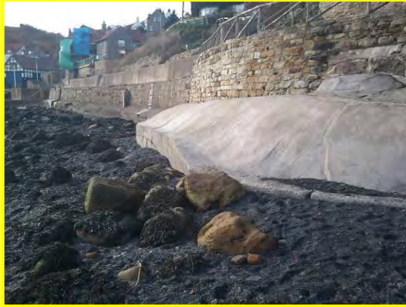
Repaired vertical cracks to toe of wall, and horizontal cracks holding, Oct 2012. (Asset Ref. 1221D901D0601C06)
