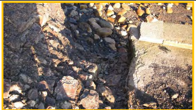
Further erosion of cliff adjacent to north end of seawall, and seawall damage since July 2013, from the top promenade, 17 th December 2013. Old concrete wall/cliff abutment now missing. (Asset Ref. 1221D901D0601C01)
