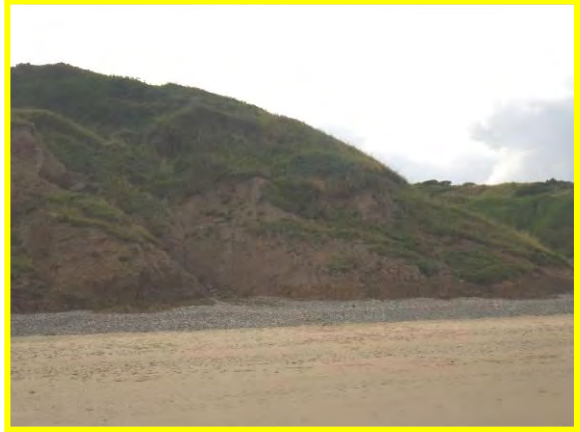
MU29/BA The small unit at Butcher Haven does not support vegetation on its lower slopes and is undergoing erosion. (Locally Active). Sept 2012
