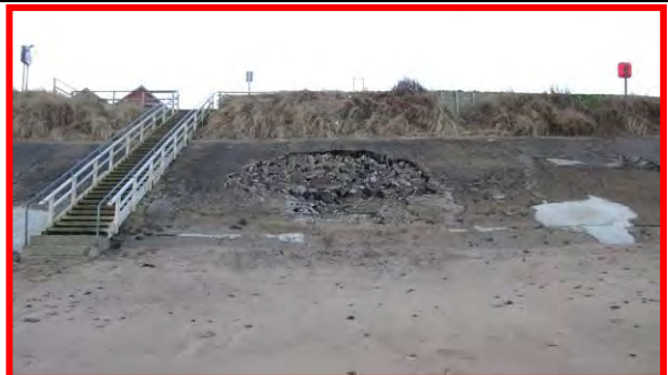
More voids forming in surface of concrete revetment, 17 th December 2013. (Asset Ref. 1221D901D0702C02)
