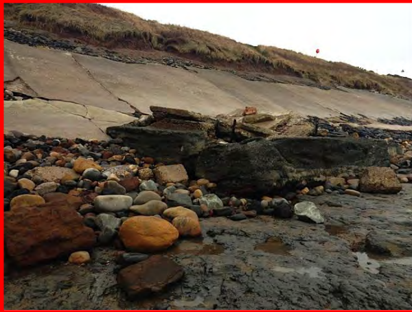
Extensive damage to revetment and the scoured beach with no sand in front of the revetment, 8 th December 2013, NYCC inspection. (Asset Ref. 1221D901D0702C02)
