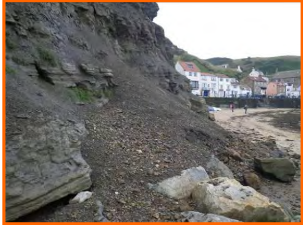
MU4/2 – There have been a number of recent failures in this management unit, which is now classed as Partly Active. Photo from Sept 2012
