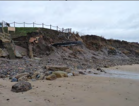
MU29/AS – Severe toe erosion and failure of steps and fences, southern end of unit. December 2013 (Partly Active).
