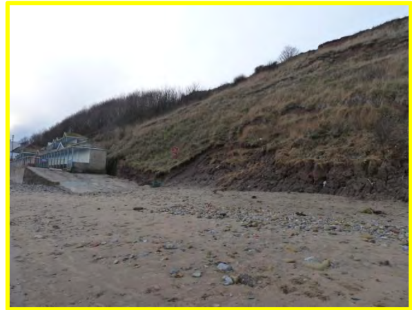
MU27/X – Some toe erosion occurring at undefended northern end of unit (closest in photo) and movement on slope (Note angle of red sign). December 2013 (Locally Active).
