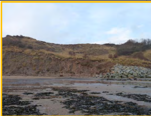
MU17/2 Recent erosion at toe and erosive features higher in cliff, December 2013 (Partly Active).
