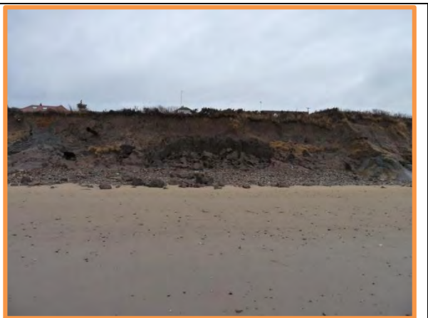
MU29/AS – Severe toe erosion including failure blocks. Note protruding pipe. December 2013 (Partly Active)
