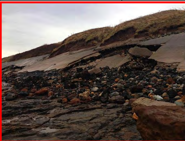
Extensive damage to revetment and cliff material above revetment. Note also the scoured beach with no sand in front of the revetment, 8 th December 2013, NYCC inspection. (Asset Ref. 1221D901D0702C02)
