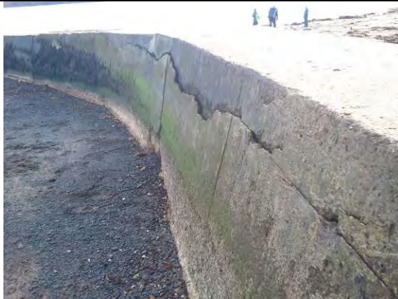
Large horizontal crack to breakwater, Oct 2012. (Asset Ref. 1221D901D0601C02)
