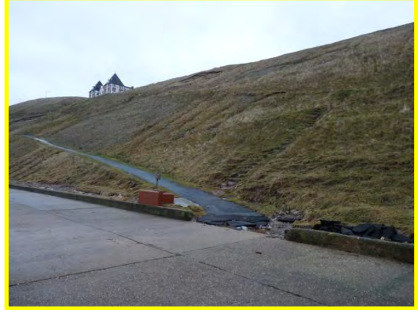
MU11/2 – Failures in upper to midslope. December 2013. (Locally Active).
