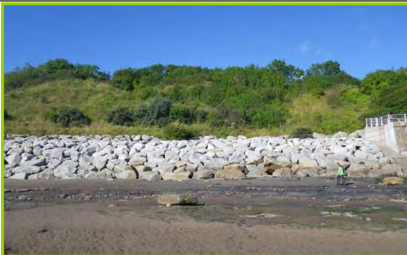
MU17/1 The defended toe and heavily vegetated slopes show that the unit has been stable (Inactive) Sept 2012
