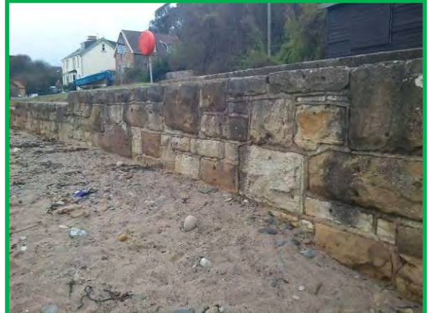
Low masonry wall at east Row Beck, north bank, Oct 2012. (Asset Ref. 1221D901D0702C03)
