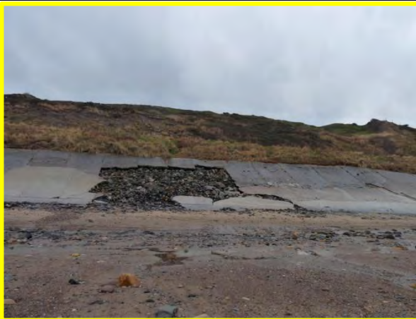
MU9/3 – Note erosive features in the upper slope as well as failure of toe defence. December 2013
