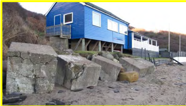
Runswick Bay sailing club concrete block defences at south end, 17 th December 2013. (Asset Ref. 1221D901D0602C05)
