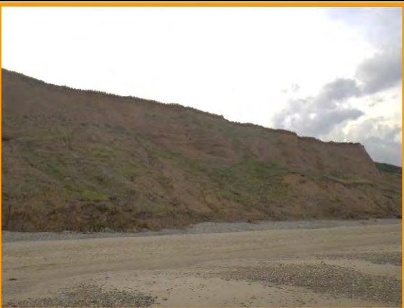
MU29/BB and BC Steeper cliffs with very common areas of intense erosion (Partly Active). Sept 2012
