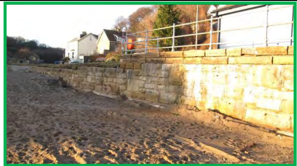
Low masonry wall at East Row Beck, north bank, 17 th December 2013. (Asset Ref. 1221D901D0702C03)
