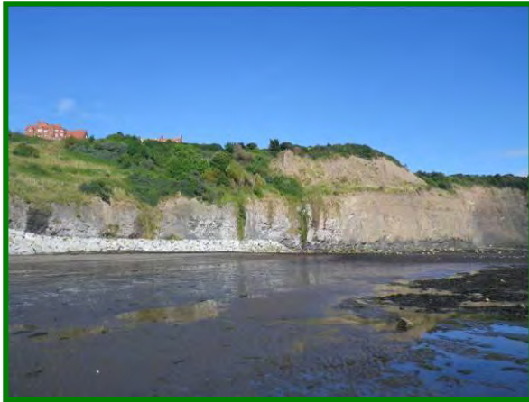
MU16/2 The cliffs have been stabilised at the toe but show some signs of erosion on their face (Dormant). Sept 2012
