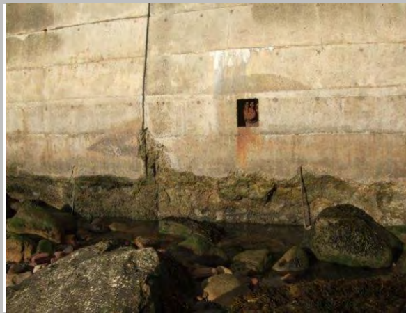
Undercutting of the northern coastal sea wall (Photo taken from 2009 report)
