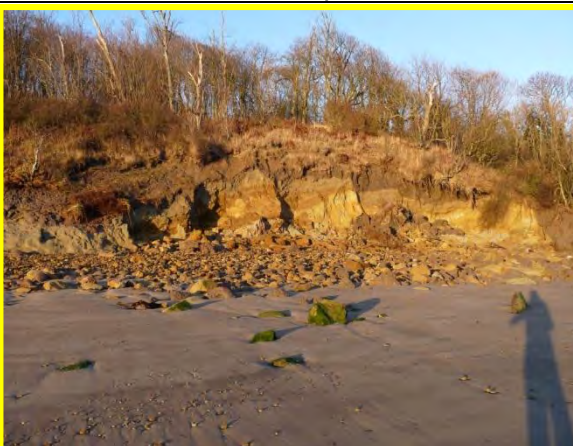
MU24/A - Toe erosion in bedrock (not in situ). December 2013. (Locally Active)
