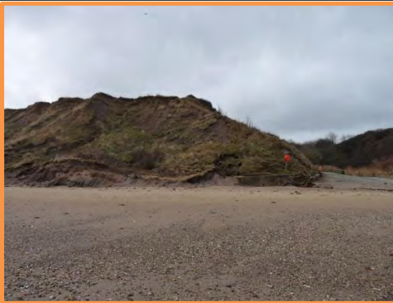
MU29/AJ – Continued intense upslope erosion and recent toe erosion/failure, particularly in the centre photo. December 2013 (Partly Active).
