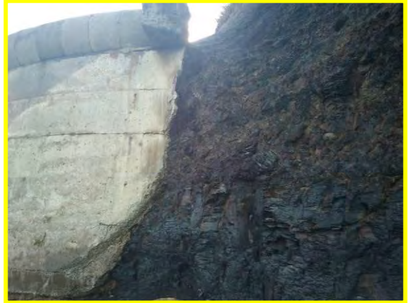
Erosion of cliff adjacent to north end of seawall, 30/10/2012 (Asset Ref. 1221D901D0601C01)
