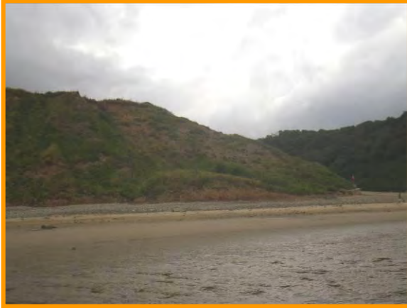
MU29/AJ Areas of intense erosion at the toe and headscarp (Partly Active). Sept 2012
