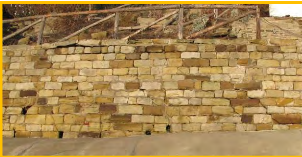
Same area as above with diagonal cracks and coping damage in wall, 17 th December 2013. (Asset Ref. 1221D901D0601C03)
