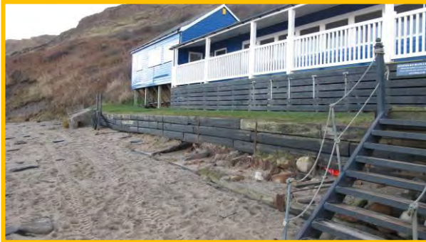
Runswick Bay sailing club timber defences at south end, 17 th December 2013. Note missing steps to beach. (Asset Ref. 1221D901D0602C05)
