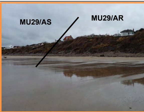
MU29/AR and AS – Substantial toe erosion throughout unit exposing drainage pipes. December 2013 (Partly Active).
