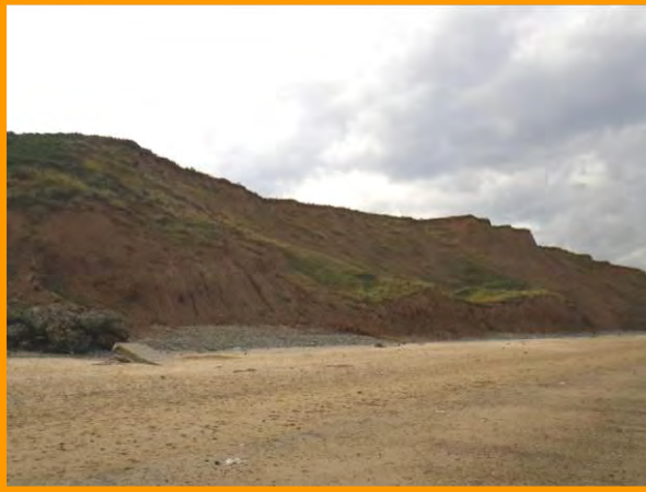
MU29/BE Headscarp and toe erosion (Partly Active). Sept 2012
