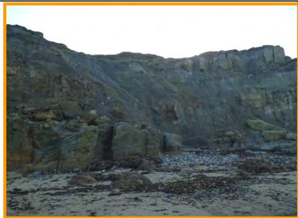
MU23/B Recent failure of the cliff (Partly Active) Sept 2012
