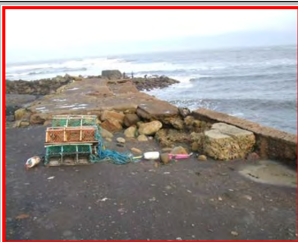
Looking at the end of the breakwater with evidence of erosion and failure in 2009 (Asset Ref. 1221D901D0502C01)
