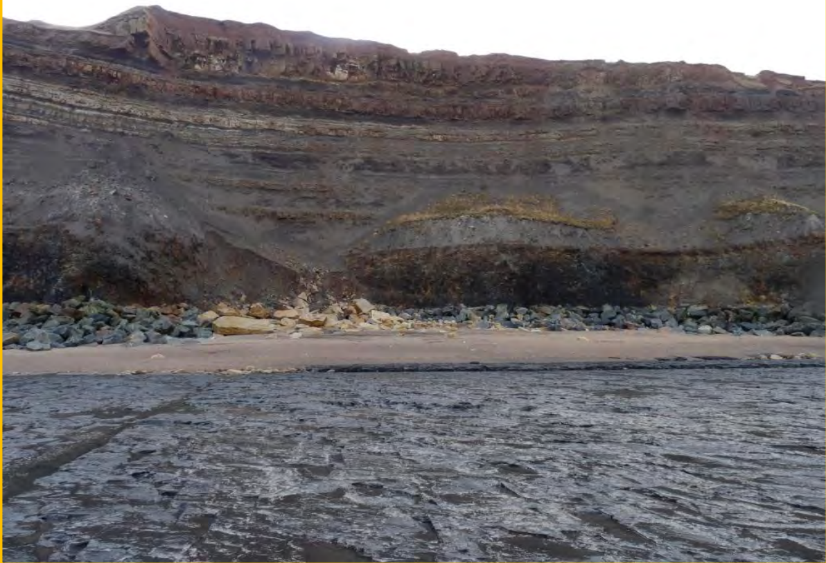
MU12/2 – Major recent rockfall and failure of lower slope/toe erosion indicating ‘Partly Active’ status is still appropriate. December 2013.
