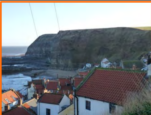
MU4/2 – Cliff behind Staithes harbour. No notable change post December 2013 surge except lack of talus accumulation. (Partly Active)
