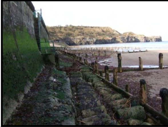
Timber toe of sea wall in a poor state - photo from 2009 (Asset Ref. 1221D901D0702C01)
