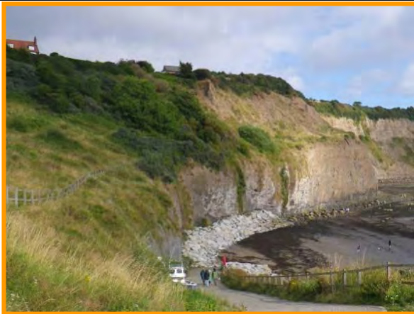
MU16/1 Cliffs below the upper part of Robin Hood’s Bay Village (Partly Active) Sept 2012
