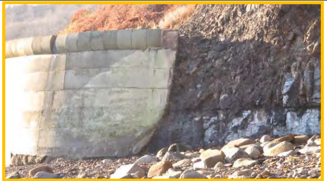
Erosion of cliff adjacent to north end of seawall, 17 th December 2013. (Asset Ref. 1221D901D0601C01)
