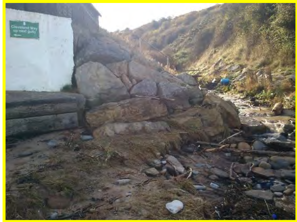
Northern end of defences at Runswick Bay sailing club, Oct 2012. (Asset Ref. 1221D901D0602C05)
