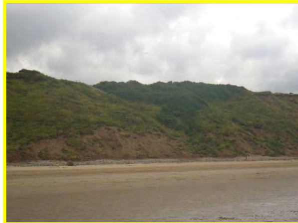
MU29/AH Heavily vegetated with toe erosion, which is severe in places (Locally Active) Sept 2012
