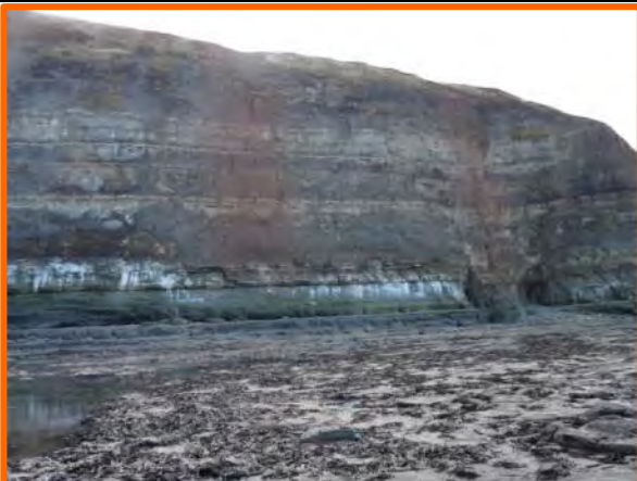
MU4/3 – Undefended cliff east of Staithes Harbour. Note red-brown ‘streaking’ on cliffs from failures in till.
