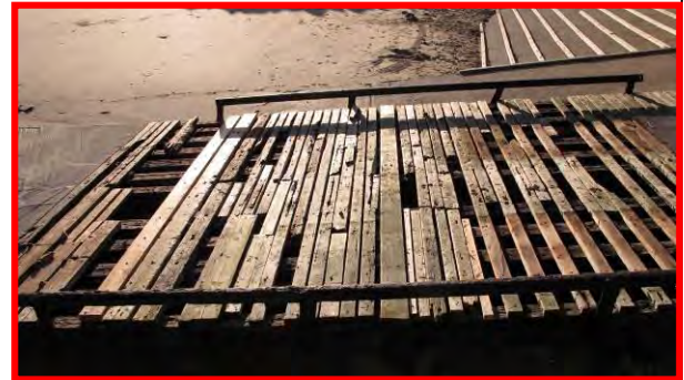
RNLI slipway damage viewed from the pumping station, 17 th December 2013. (Asset Ref. 1221D901D0601C04)
