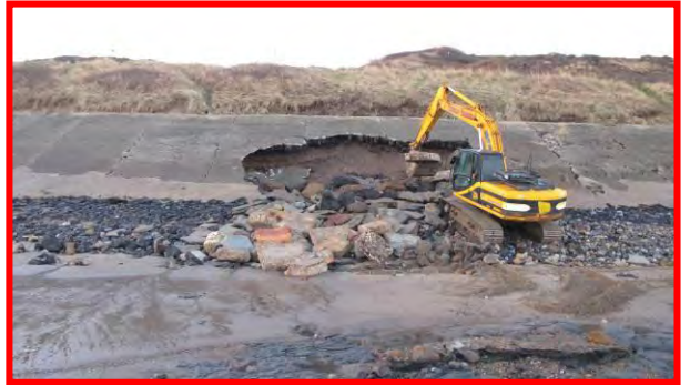
Temporary repairs to revetment being carried out on 17 th December 2013. (Asset Ref. 1221D901D0702C02)
