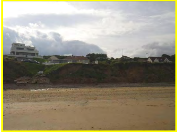
MU29/AS Continuing mudslide activity and toe erosion at Flat Cliffs (Locally Active). Sept 2012
