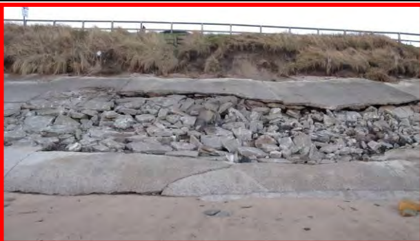
Extensive damage to revetment temporarily filled in, 17 th December 2013. (Asset Ref. 1221D901D0702C02)
