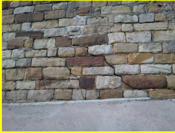
Diagonal cracks in wall. Oct 2012. (Asset Ref. 1221D901D0601C03)
