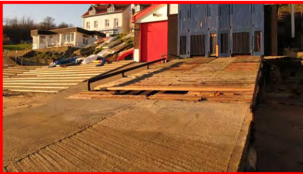
RNLI slipway damage, 17 th December 2013 (Asset Ref. 1221D901D0601C04)
